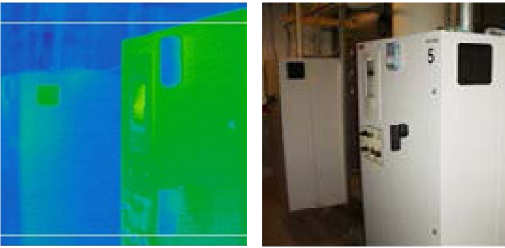
Figure 4 Thermographic and visual image documenting increased heat of VFD P-5 after fan removal.
