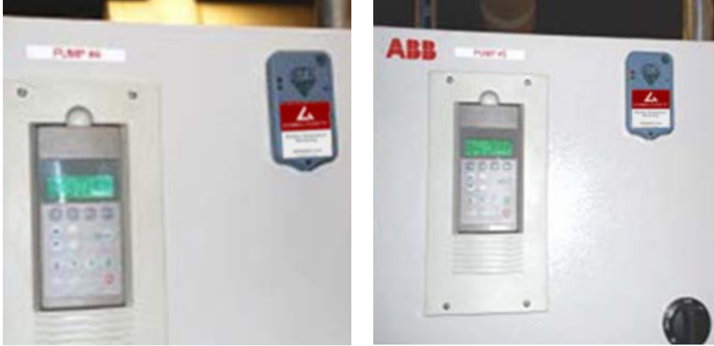
Figure 1 Delta T Alerts installed on VFD's P-4 and P-5.
